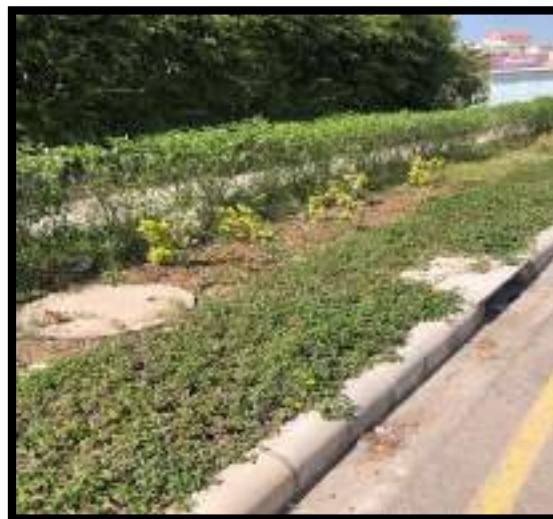
Photographs of rain water recharging pit provided within project premises
